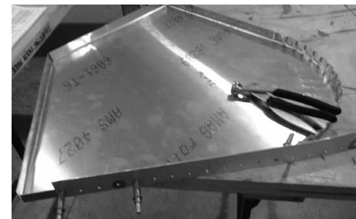
The first challenge is building a 16 foot long work table to cradle the floats as you start construction. At 15' long, the Zenair 1450# floats require a 3' long piece be fastened to a standard 4x12' sheet of 6061. The bulkheads share the same profile, but vary in height.
