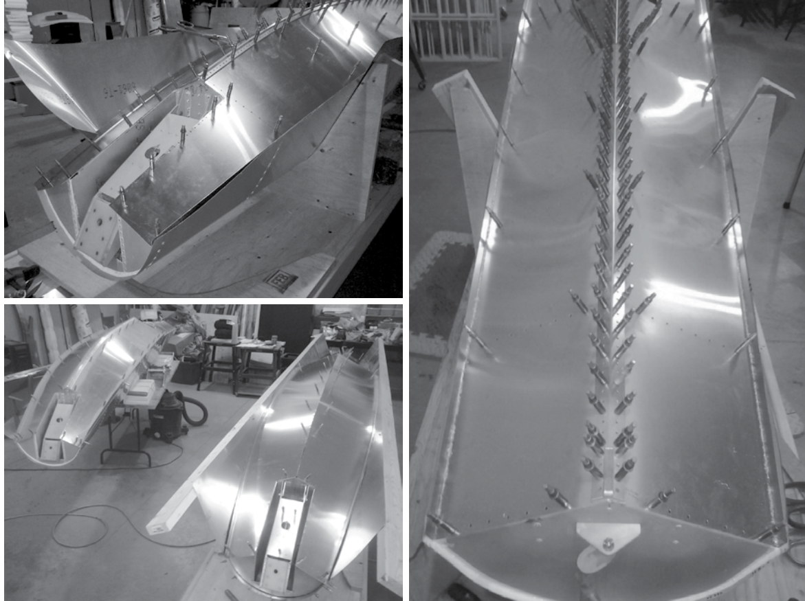
Top left: Once the bottom skins are positioned and held with clecos, the side skins can be trimmed back to reveal the true shape of the floats. Lower left, once the first float was finished to a point where it could be safely moved, I started the second float. Right: since the keels take most of the abuse when a float touches the bottom of a lake or river, they are made from a heavy extrusion that protects the float skins.
